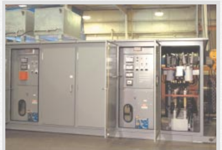
Control and Control Power Compartments
