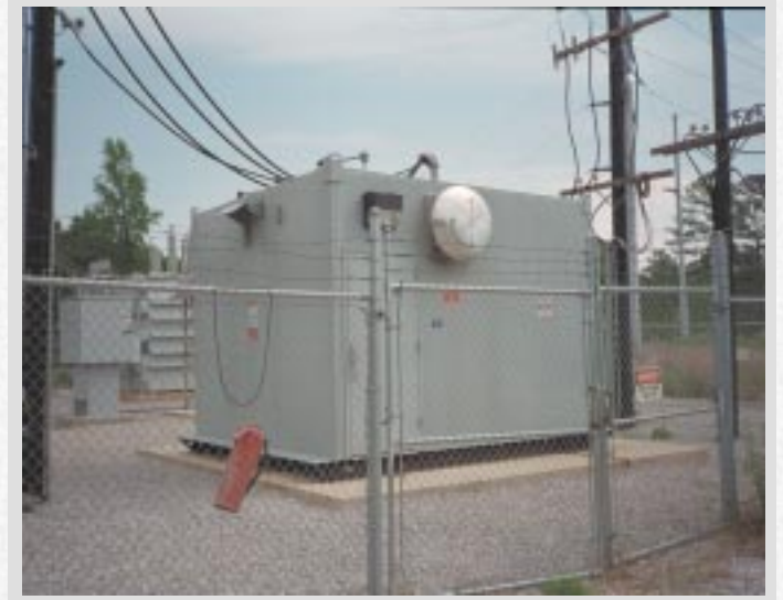
Padmounted Switchgear Substation
