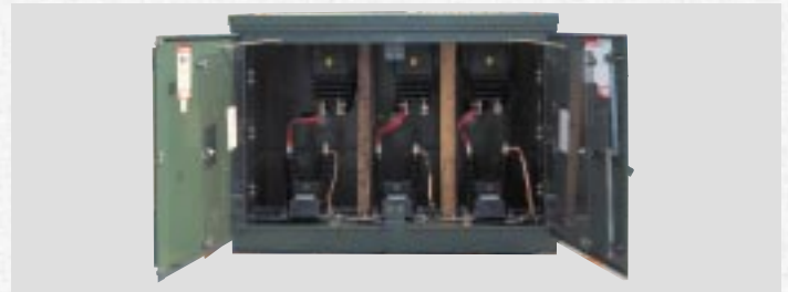
Metering Transformer Compartment
