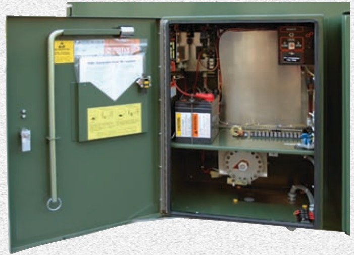
Figure 3. FP Motor Operator. The reliable FP motor operator contains the many features for local automatic operation, including a long-life battery and charger for power to DC circuits.
