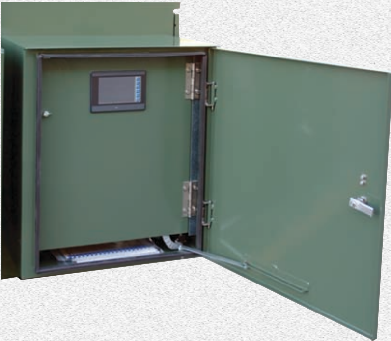
Figure 2. Low-voltage control compartment containing the FP automatic-transfer micro-processor control.
