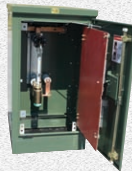
Fuse Compartment Interior With Hinged Barrier Secured Open and Fuse Closed and Latched
