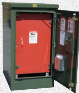
Fuse Compartment Interior With Hinged Barrier Bolted Closed
