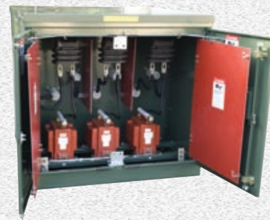
Metering Transformer Compartment With Barriers Secured Open
