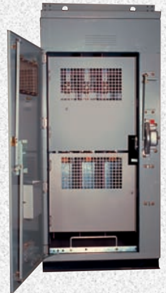
Open Door View of Switch/Fuse Bay Showing Internal Screen
