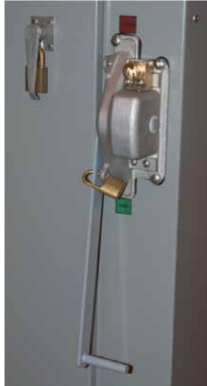
Figure 18. Key interlocks on manual switch-operating handle to guard against possible undesirable paralleling and to prevent opening the door unless downstream switches are open.
