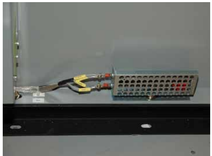
Figure 2. Strip heater is mounted behind a perforated sheath on side wall of enclosure.
