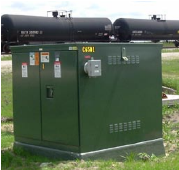
Figure 9. Padmounted capacitor banks provide an esthetic installation, avoiding overhead clutter.
