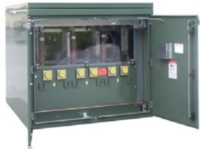
Figure 3. Incoming connections are through bushing wells that accommodate inserts and elbows (not furnished) to the protective devices, which in this installation are current-limiting fuses visible through the polycarbonate barrier.
