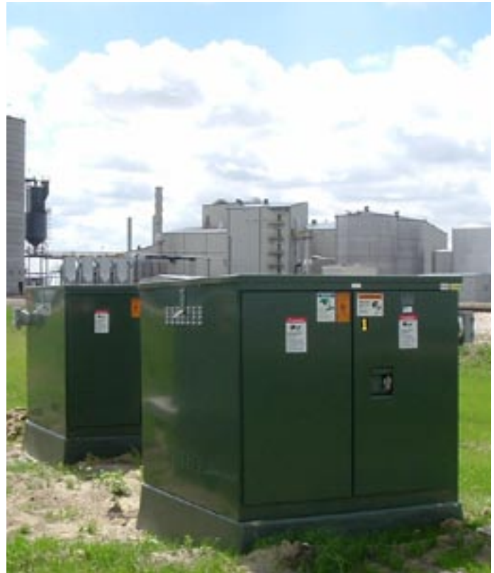
Figure 10. Padmounted capacitor banks provide power factor correction near industrial loads.
