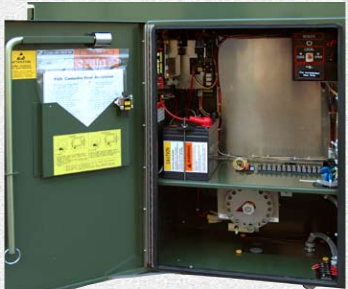
Figure 2. Motor operator provides space for an RTU, radio and antenna, power supply, control power source and associated components.
