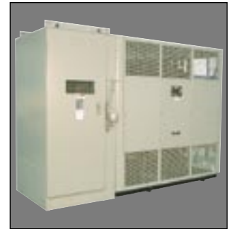
Unit Substation Transformer with Primary Switch
